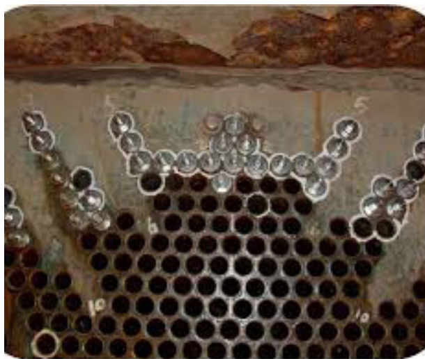
Figure 3 - Leaking Tubes are Plugged Out of Service
