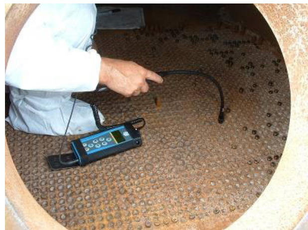
Figure 7 - Finding Tube Leaks with SDT Ultrasound
